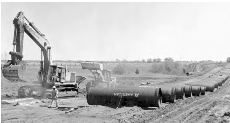
60" AMERICAN Fastite® Joint Ductile Iron pipe being installed as a water transmission main.
