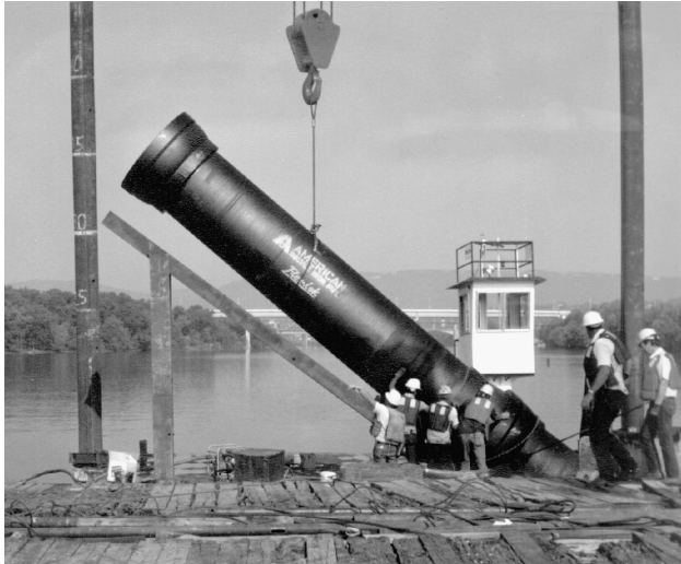
48" Flex-Lok Pipe being positioned for assembly. The ramp attached to the barge is used as the assembly platform, and as the joints are made, the barge is moved forward, allowing assembled piping to slide into the water.
