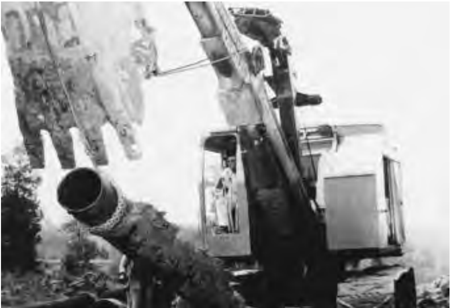
Cast Iron Pipe – being replaced by a larger main – is taken up after years of service for installation in another location for continued service.
