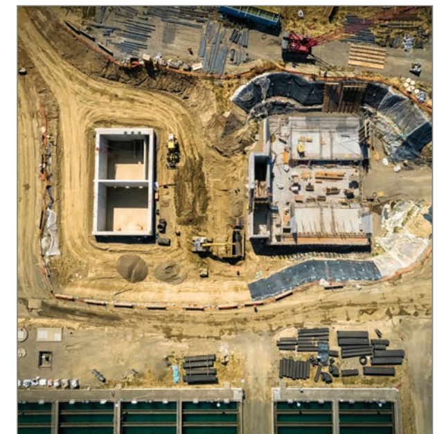
Overhead view of water treatment plant utilizing AMERICAN Earthquake Joint System.
