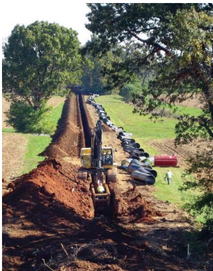
Figure 3. A 24-inch (600 mm) diameter cement lined ductile iron transmission line being installed.
