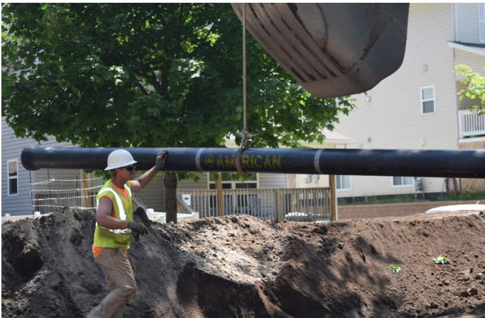
AMERICAN Ductile Iron Pipe with zinc coating being installed by Danner Inc. in Saint Paul, Minnesota.
