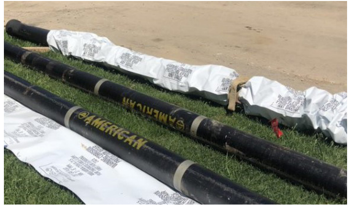
SGP Contracting Inc. prepares AMERICAN Ductile Iron Pipe with zinc coating and V-Bio polyethylene encasement for installation.
