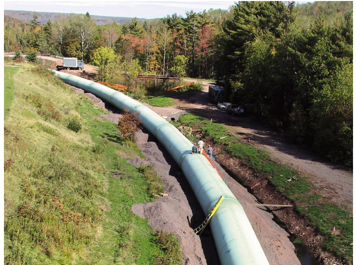
Figure 10. An upper peninsula Michigan penstock by AMERICAN SpiralWeld.
