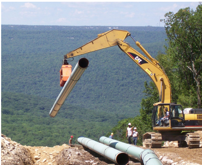
Figure 9. AMERICAN Steel Pipe ERW line pipe being installed to deliver natural gas.
