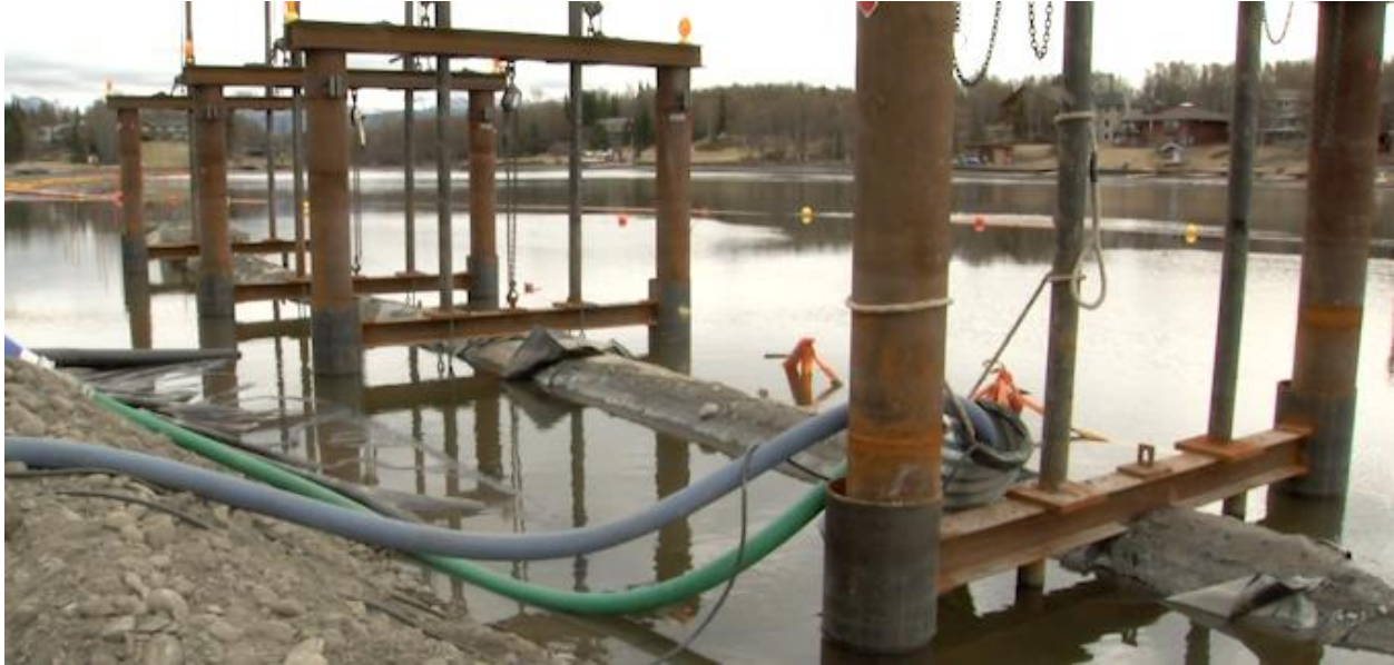
Figure 4. A stabilizing assembly driven into the lakebed to hold the ductile iron piping in place after the ice had melted.
