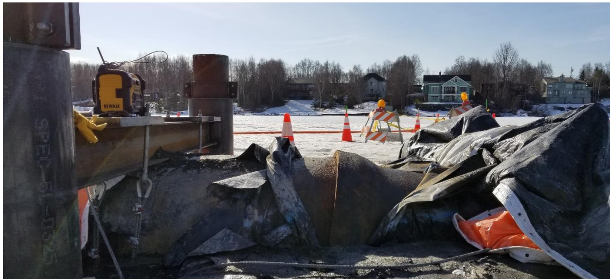
Figure 9. The exposed most-severely deflected joint showing condition of the traditional polyethylene encasement and the peen pattern of the pipe surface after 29 years beneath the lakebed.
